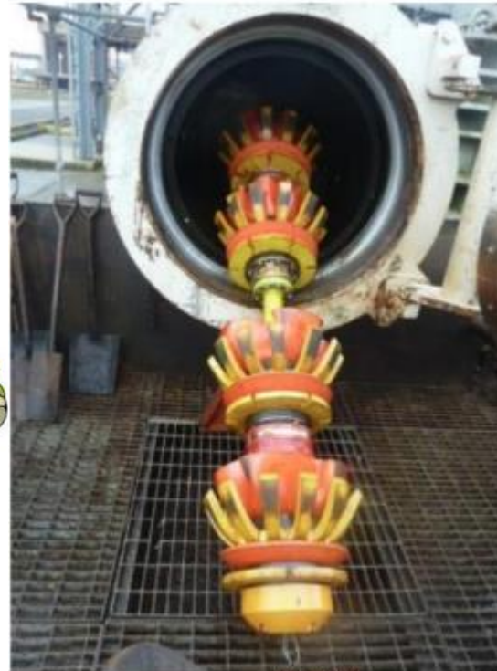
16/24E pig received at Teesside 34" pig receiver
